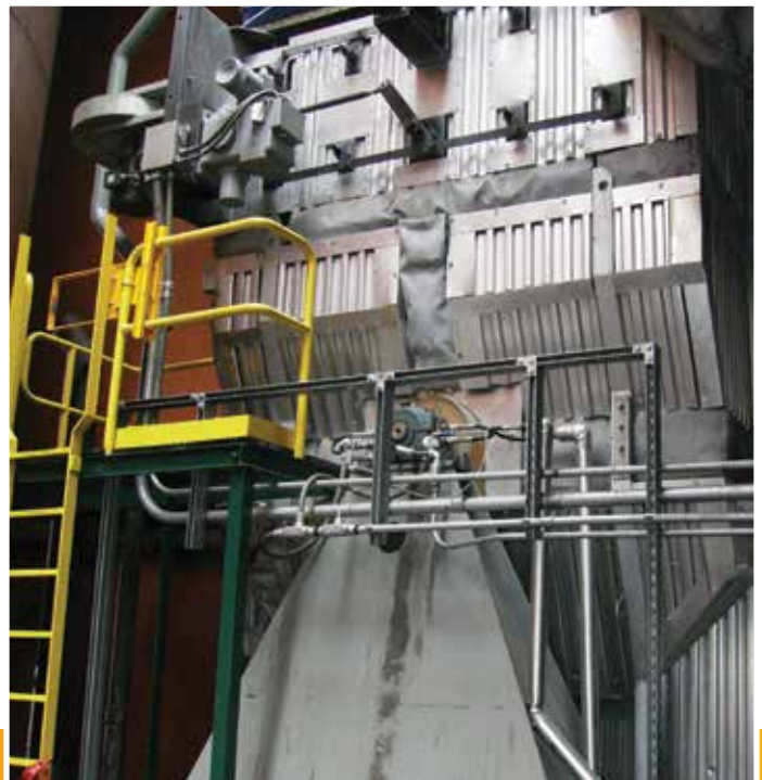
RECIRCULATED OVER FIRE AIR - USA DRBS 2316 SR.47 SWSI, Radial Bladed Draft Fan, Arrangement 7B Performance: 92,000 cfm, 29.0 in wg SP, 650 F° Density 0.034 lb/ft 3 , 1190 rpm and 602 BHP
