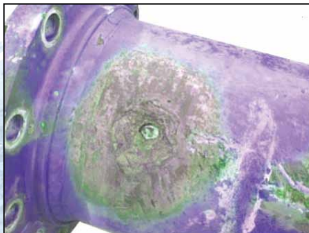
Corrosion of the vent hole area following permeation and no particular corrosion protection
