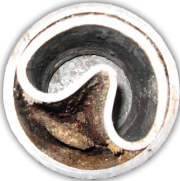
Cut steel pipe showing PTFE lined collapse through blocked vent holes
